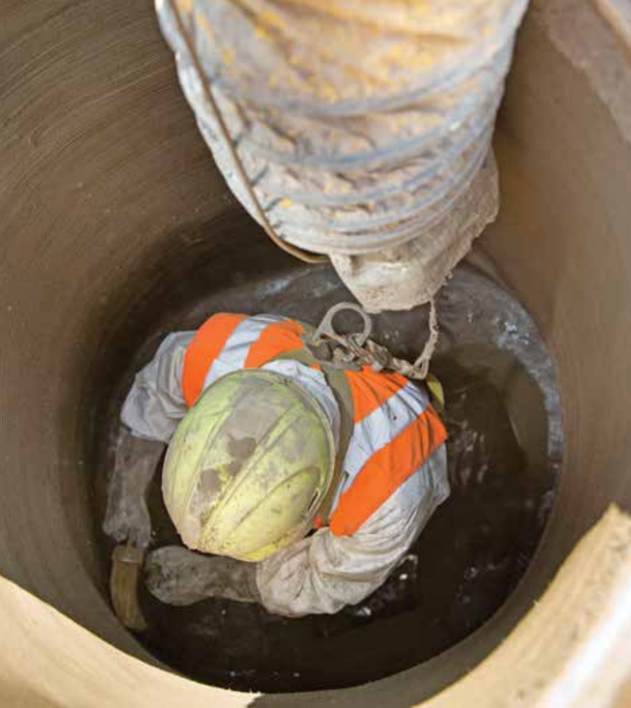
<< Felipe Servin brushes the final coat of Strong Seal MS- 2C cement liner inside a manhole.
