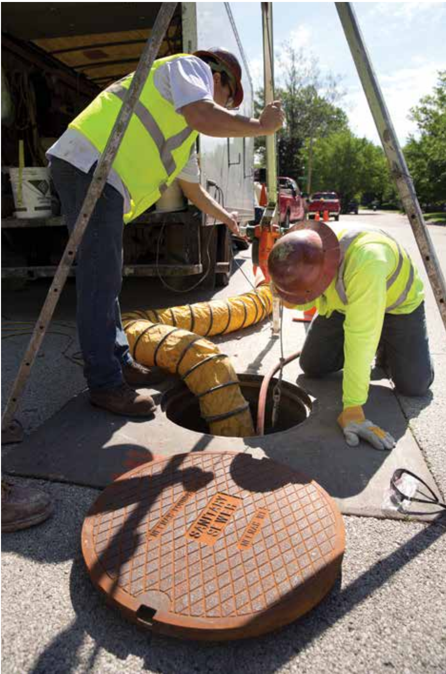
◀◀◀ Brett Vallow (left) and foreman Michael Walsh visually inspect a cement liner, measuring vertical footage for build quantity.
