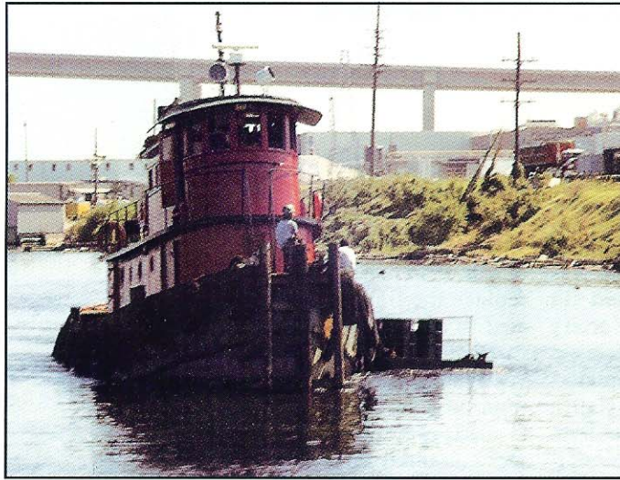
Work tug transporting chemical grout containers to work platform. All of the work on this project was done from floating platforms secured parallel to the pipeline.
