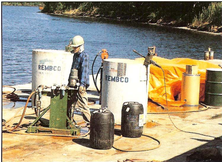
Material proportioning equipment in front of the grout (left) and water supply tanks. The grout was injected every two feet.
