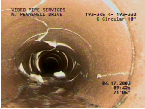
Figure 1 Structurally Compromised Pipe
