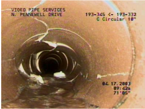
Figure 1 Structurally Compromised Pipe
