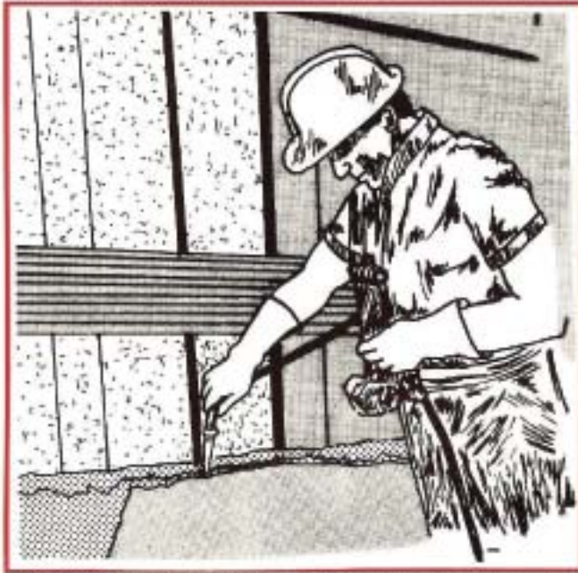
Flushing the joint prior to injecting PUR in tunnel joint with active water leakage.
